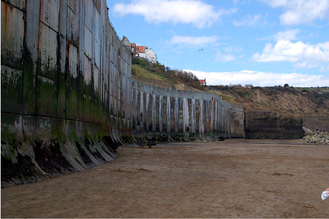
Figure 17: The Sea Wall at Robin Hoods Bay, North Yorkshire, North East England – notice the lack of any form of nature as the intrusive sea wall destroys any potential ecosystem environment
