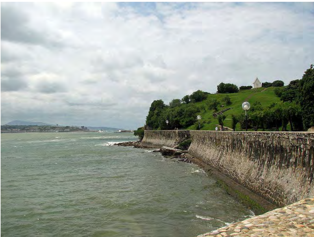
Figure 18: The Sea Wall at Saint Jean de Luz Bay, South West France.
